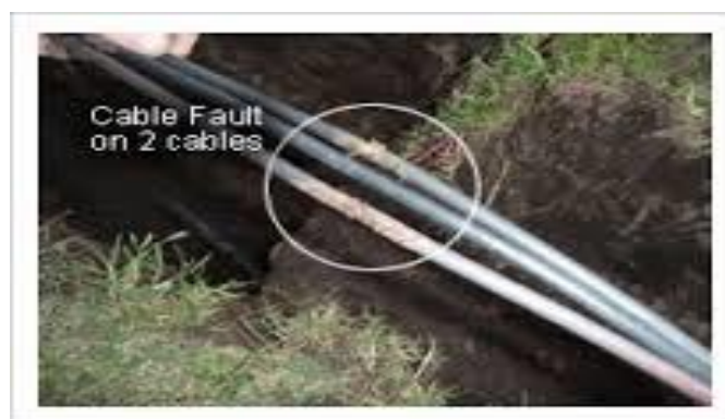
Fig1: Underground cable fault
