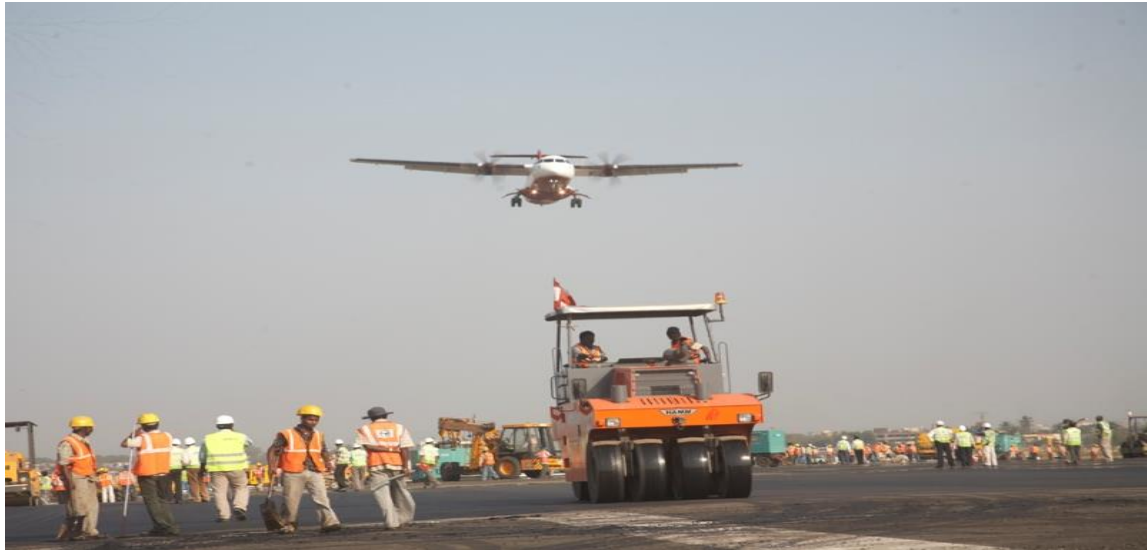
Fig-1.2- Concrete Finishing Layer of concrete with Concrete Paver in HIAL runway
