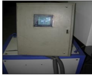
Figure2. Multifunction meter for power consumption
