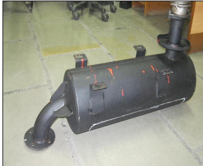
Figure 4: Diesel genset silencer
